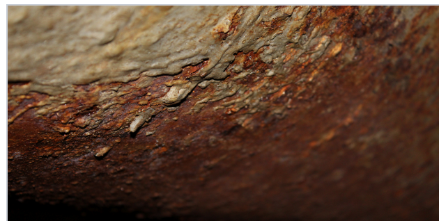
What the gaps hide: coating disbondment and active corrosion on an in-service line.
