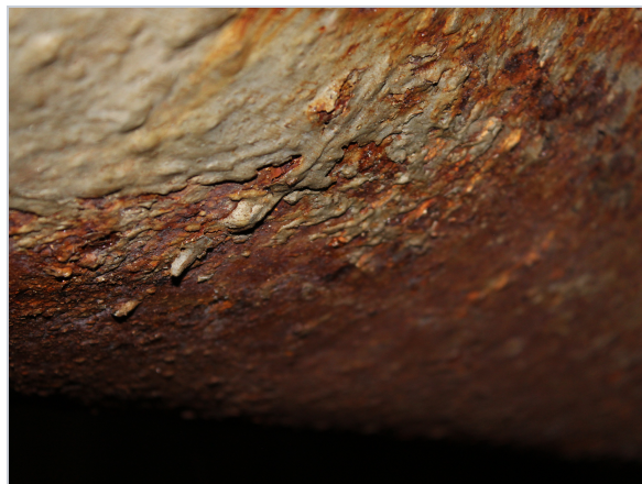
Coating disbondment and external corrosion — visible at the surface, but the wall behind it is the real question.
